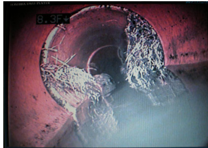
Tree roots can cause clogs and leaks
