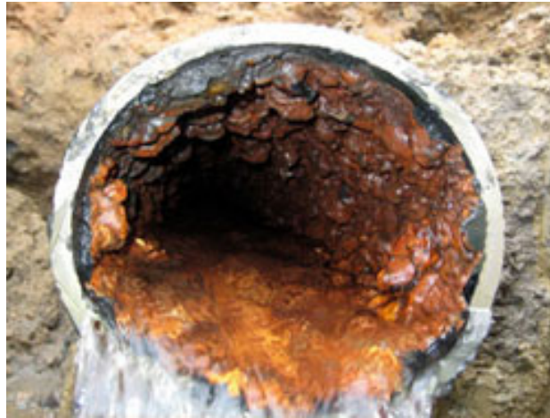
Cast iron pipe with scaling
