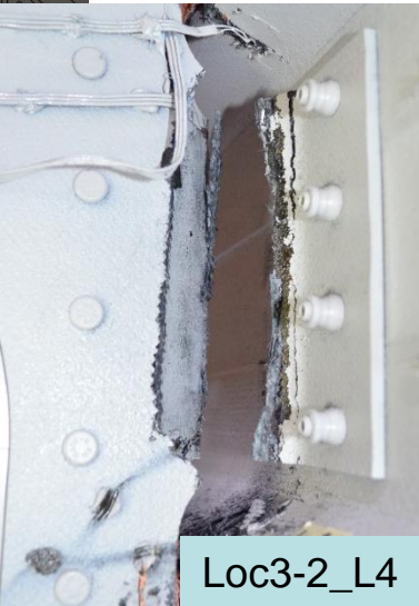
Second crack on shear tie
