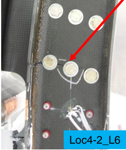
Passenger floor beam crack
