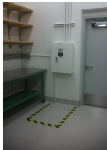
Figure 14: Clear Space Around Electrical Panel
