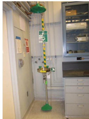
Figure 13: Eyewash Shower in Lab, Good Location
