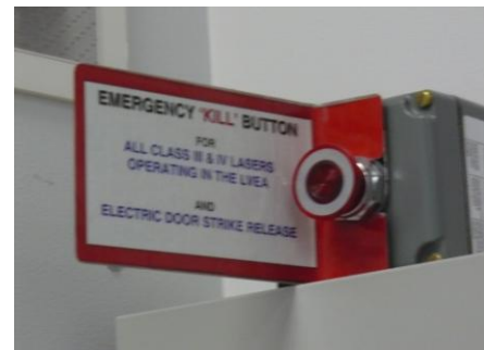
Figure 3: Labeled Emergency Stop
