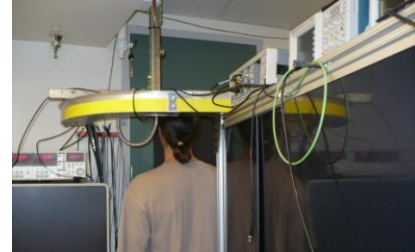
Figure 10: Cable Tray too Low
