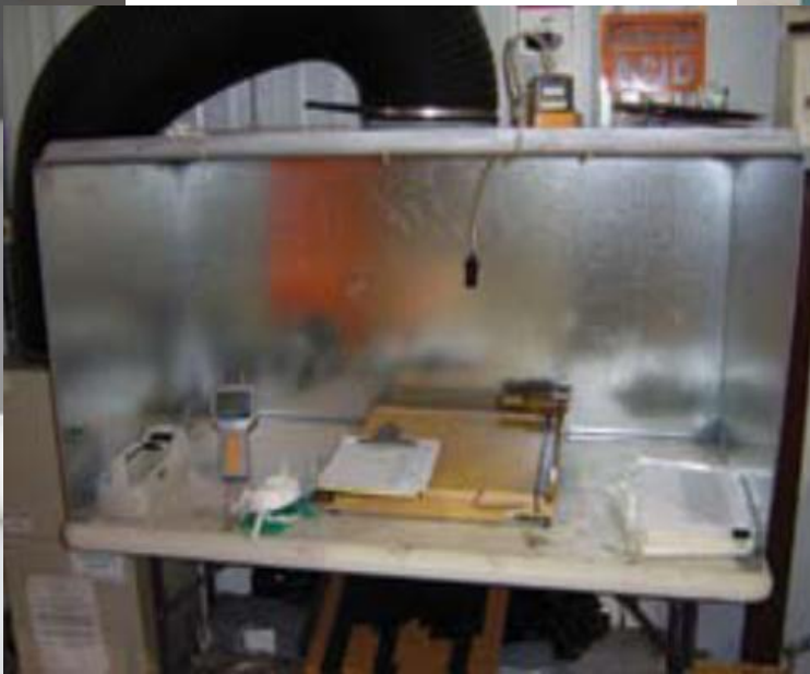
Ventilation, fume hood, filters
